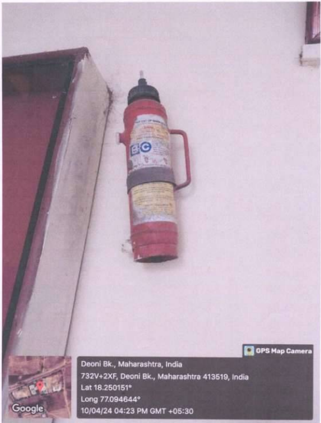
Fire Extinguisher in college campus
